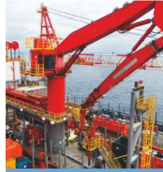
PLATFORM CRANES AND SHEAVES
